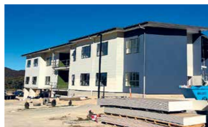
■ Above, Wattle Apartments were officially opened on 12 July. Left to right: Gary Edwards, Peter Russo MP, Hon. Mick de Brenni, Frances Paterson-Fleider and David Swain. Below, construction at the new Stanthorpe aged care service.
